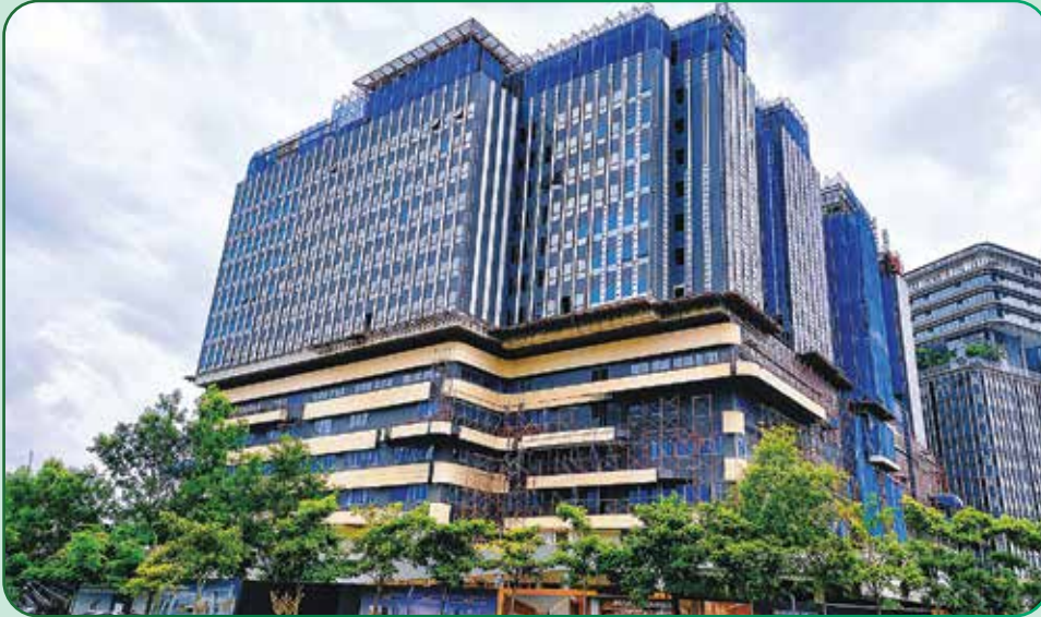
KL International Hospital project under construction (approximately 75% completed), illustrating the importance of managing construction activities responsibly within an urban environment.
