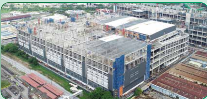
Logistics Hub – Plot B development under construction (approximately 73% completed), reflecting the Group's commitment to delivering high-quality and reliable built environments.
